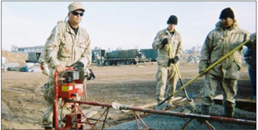
BUILDING IRAQ — Arlan Williams (left) of the University Police Department mans a concrete screed while on deployment with a team of military reservists in Taji, Iraq, where he helped build a base to eventually turn over to the Iraqi army. He served with the Red Horse unit, an acronym for a rapid deployable heavy operations and repair squadron. They built roads, wells, sanitary systems and other public works while abroad. Williams, a Commerce resident, recently returned to civilian life.
